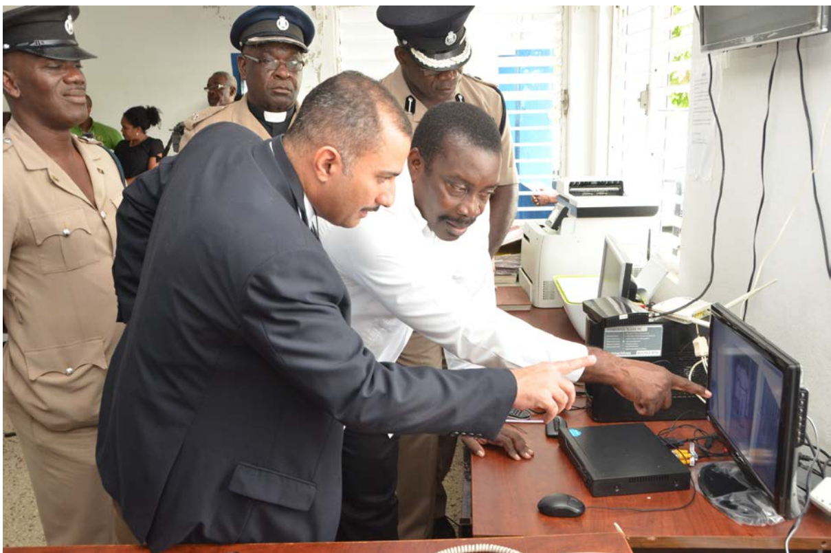
National Security Minister, Hon. Robert Montague with donor, Managing Director of Quest Security, Joseph Dibbs examining the newly installed CCTV system at Islington Police Station in St. Mary. Looking on are (l-r), Commanding Officer for St. Mary, Superintendent D. Powell, Station Chaplain, Rev. Lenford Newell and ACP Fitz Bailey in charge of Area 2.
